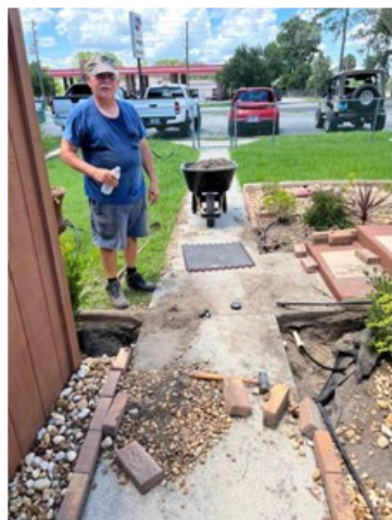
Our beloved, Bruce Russell overseeing an outdoor watering system installation for the church flowers and plants
