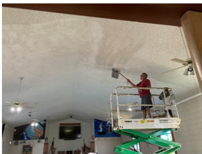
All the ceilings inside of the church were scrapped to removed the popcorn texture.
